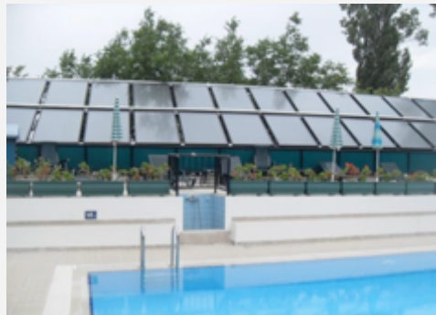
Solar pool heating systems
