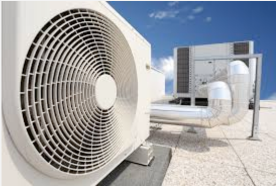
Air conditioning system
